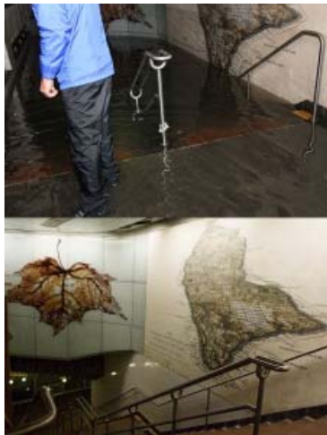
Stairs in the South Ferry station during Sandy (above) and today (below) photos: Donna Ferrato (bottom), courtesy of Tom Abdallah (top)
