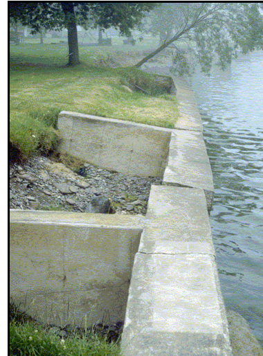
Deteriorated erosion control structures provide little or no long-term protection to shoreline property.
