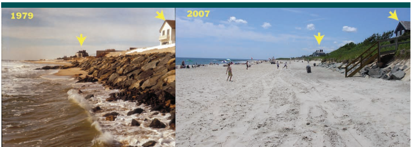
Figure 24. In stable areas with an adequate sand supply, studies over the last thirty years have shown shore parallel structures like this rock revetment can provide erosion protection during severe storms without adversely affecting natural beach building processes. (Arrows indicate the same houses in the two photos for reference.) (2007 Photo: M. Slattery)
