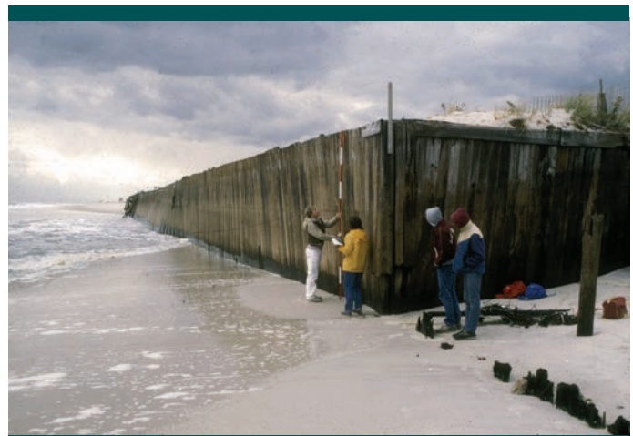
Figure 25. In areas experiencing chronic recession, shore parallel structures like this bulkhead can prevent the landward migration of the shoreline eventually resulting in the loss of the dry beach. (Photo: H. Bokuniewicz)
