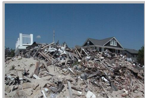
Destruction from Sandy in Mantoloking, New Jersey. Credit: New Jersey Sea Grant
