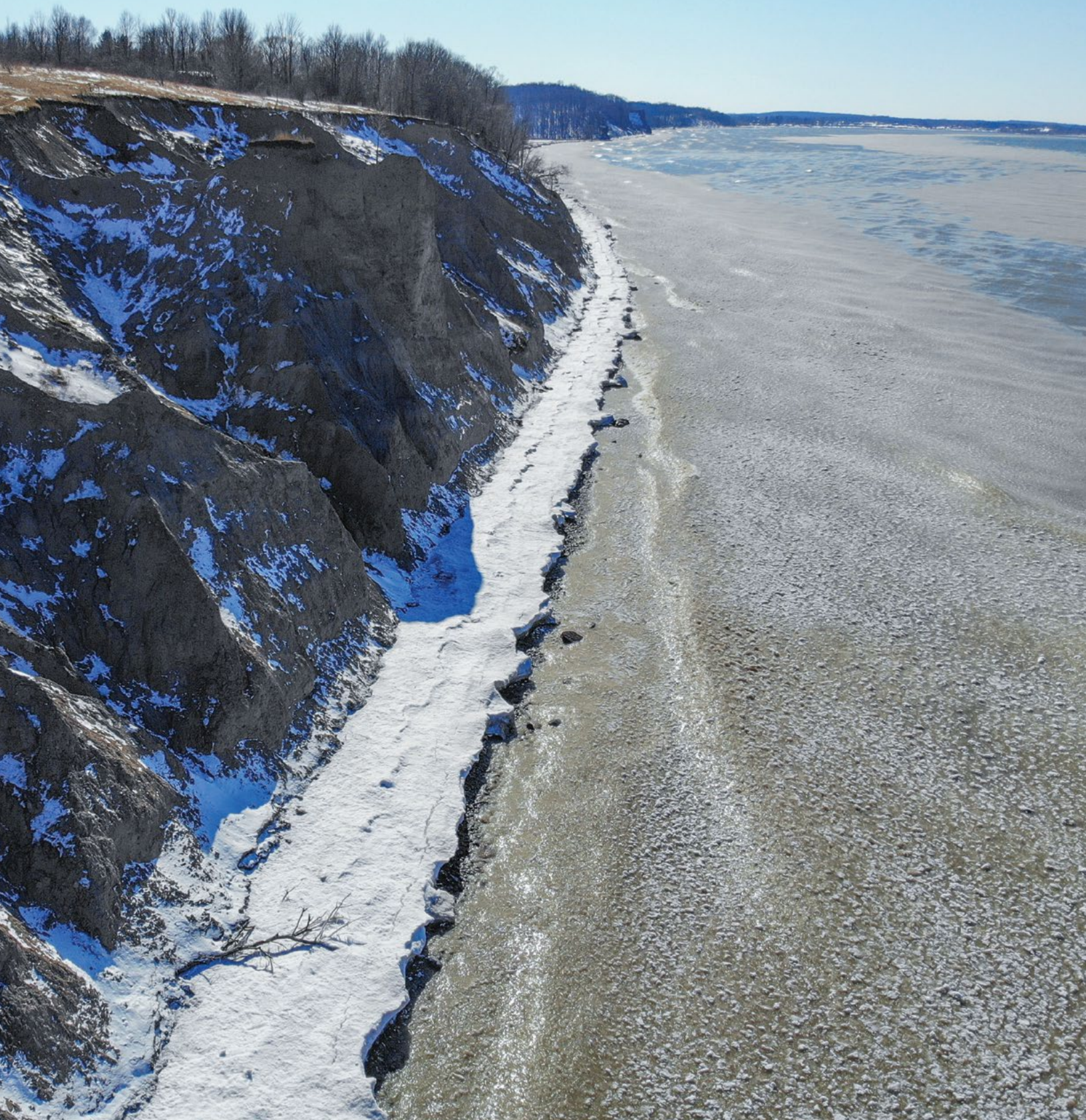
▲ Drumlins along the southern shore of Lake Ontario form steep, unconsolidated bluffs that erode rapidly in times of high water and intense wave action. Lack of shoreline ice during the winter exacerbates this process, first starting at the toe of the bluff and causing slumping further up, causing large chunks of bluff to erode at a time. Bluffs can be difficult to manage for erosion, but a combination of slope reduction (terracing), toe protection and revegetation can improve the stability of these features. Photo by Roy Widrig, New York Sea Grant.
